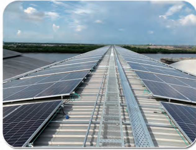
1MW SFS-WW Walkway mount System (Thailand)
