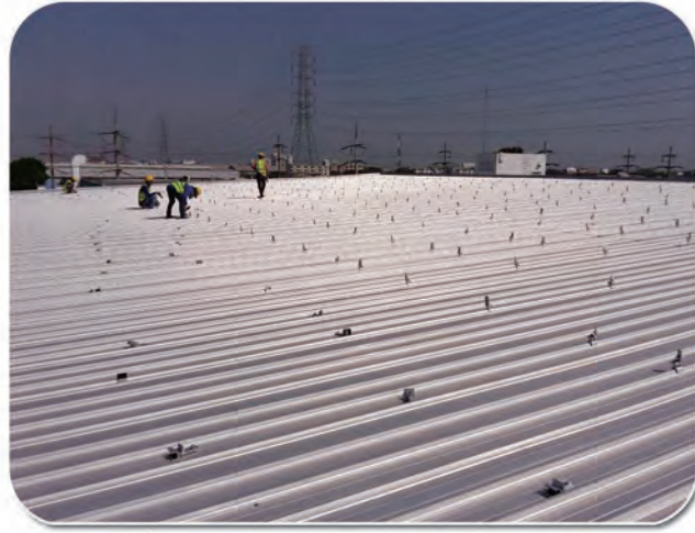
1MW SFS-PR-01 Tin Roof clamp mount (Thailand)
