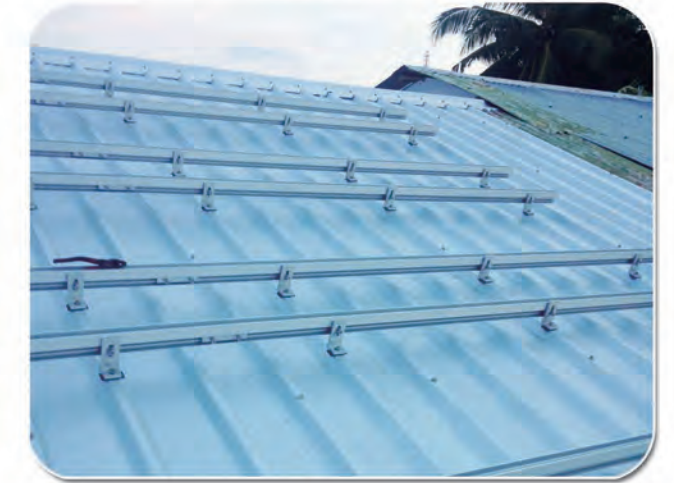
300KW SFS-PR-01 Tin Roof Mount(Philippine)
