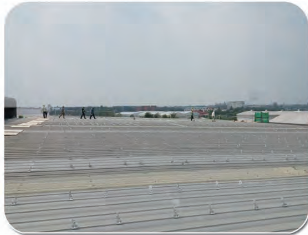
2.5MW SFS-PR-01 Tin roof clamp mount(Thailand)
