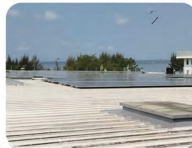
900KW SFS-PR-01 Tin roof solar mount (Vietnam)
