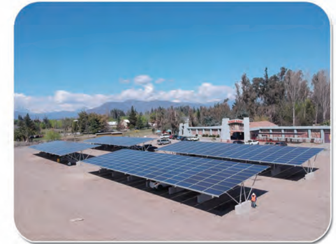
500KW SFS-CP-03 Commercial Carport mount (Chile)
