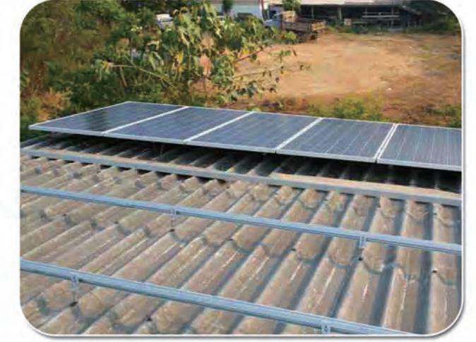
500KW SFS-PR-01 Asbestos Roof Mount(Thailand)
