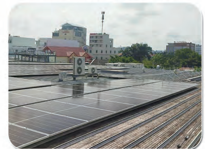
900KW SFS-PR-01 Tin roof solar mount (Vietnam)
